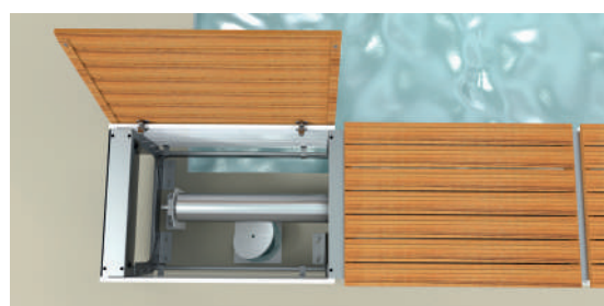
Access to the skimmers and mechanical parts
